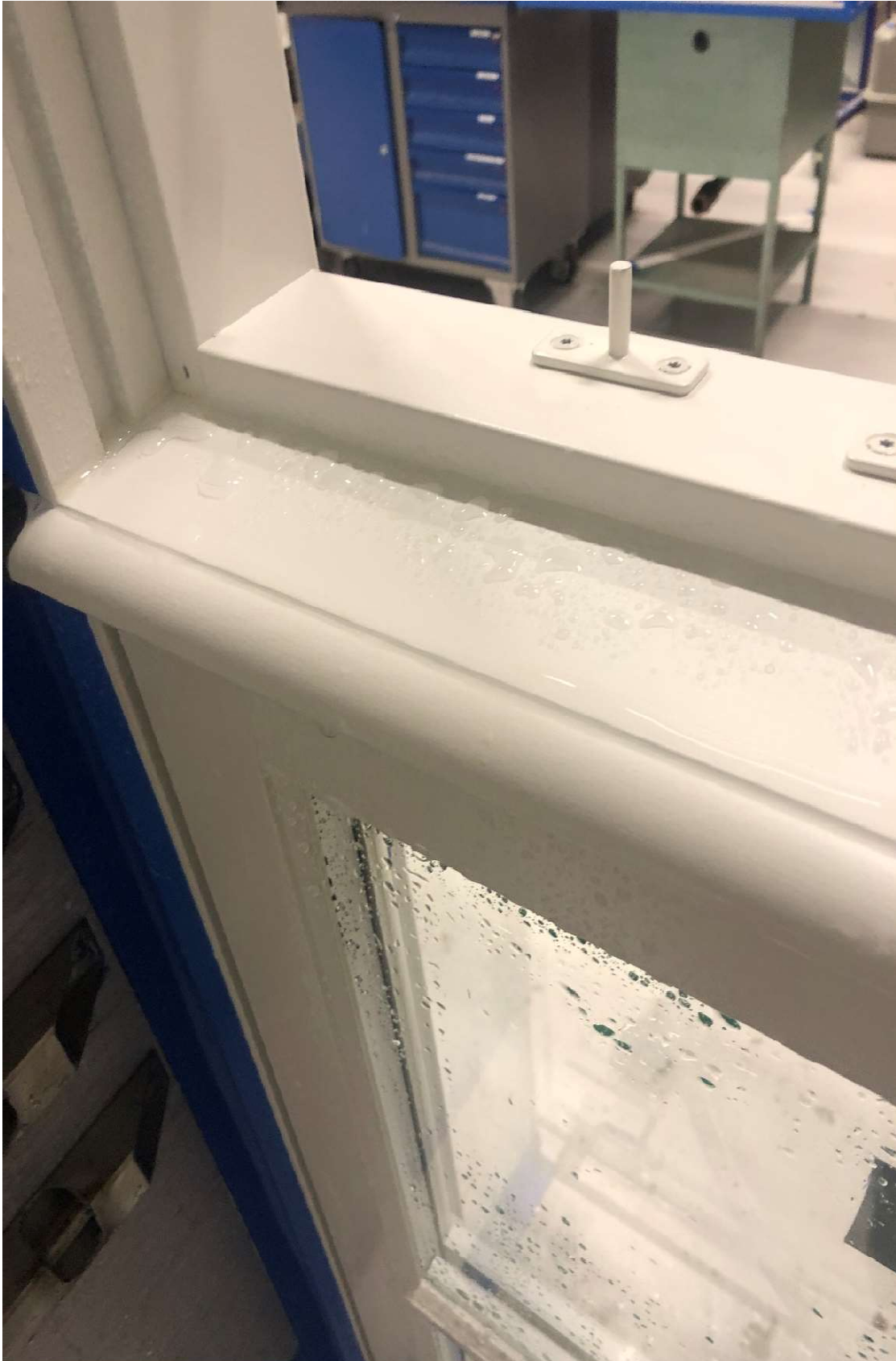
Figure 2: View of the horizontal middle post frame member after watertightness test up to 1200 Pa.
