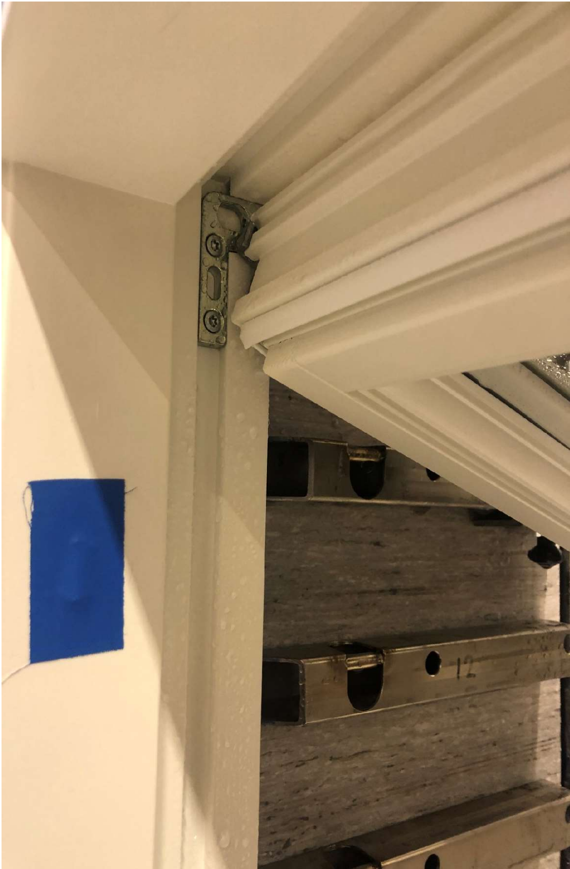
Figure 3: View of the upper horizontal frame member after watertightness test up to 1200 Pa.
